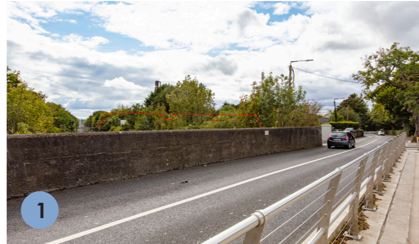
1 Enhanced bridge over the Dublin-Belfast railway. Scheme is located left, as outlined in red.
